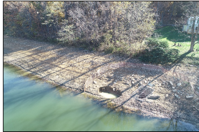
Figure 3. Sinkhole Development Along Shoreline
