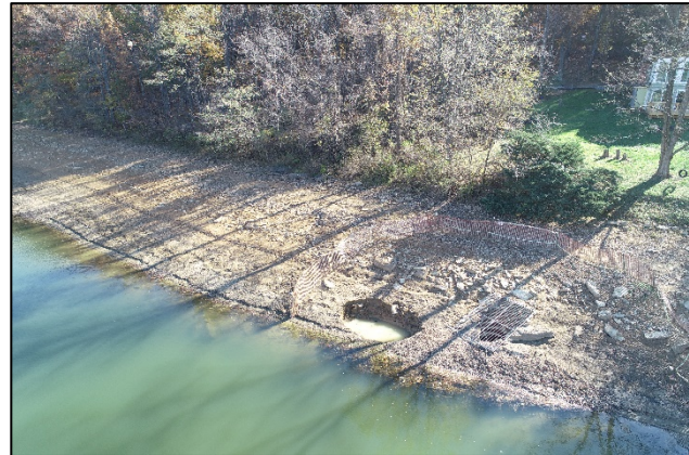
Figure 3. Sinkhole Development Along Shoreline
