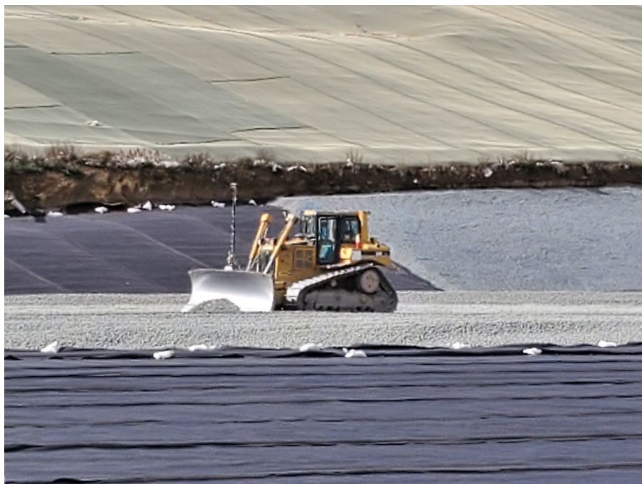
Contractor is nearing final completion of MSW Cell 3A, an eleven acre area that is being prepared for future placement of solid waste. This photo shows a dozer placing the one foot layer of leachate collection stone in the bottom of the new cell.
