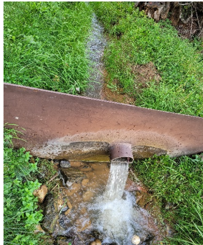
(Point where the leak is measured)
