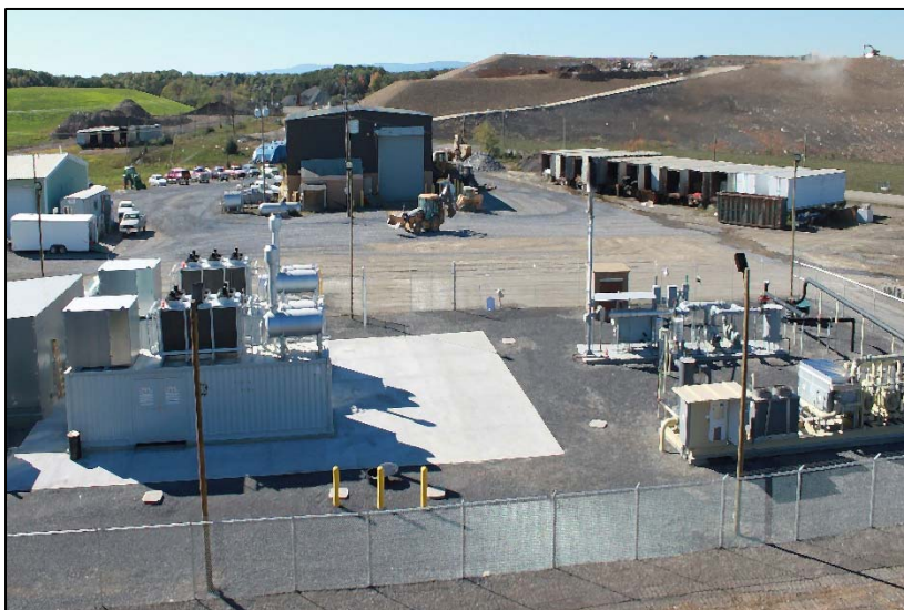
Landfill Gas to Energy Plant
