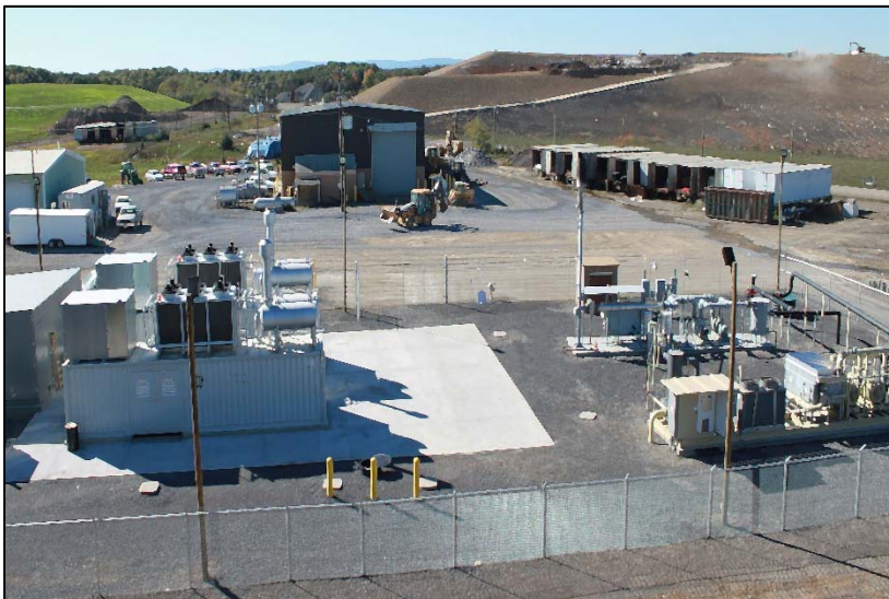
Landfill Gas to Energy Plant
