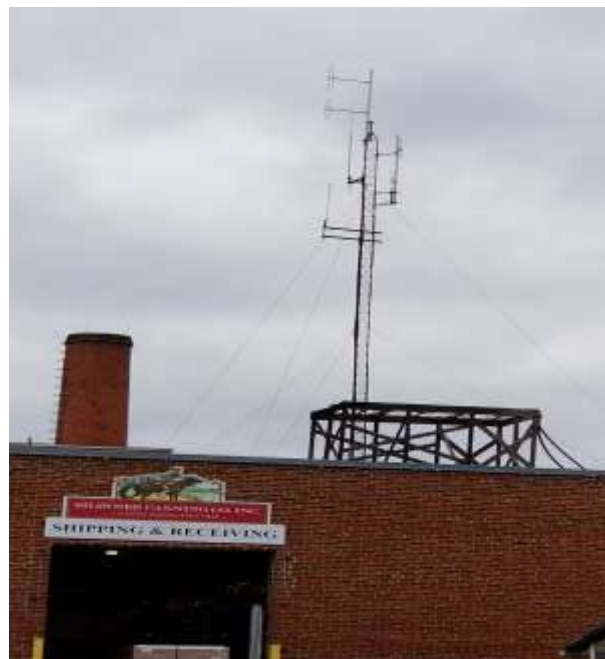
Figure 9: Cross-Junction antenna at cannery building
