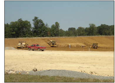
Photo courtesy of Gloria Puffinburger Clay being rolled into new CDD cell, September 2012.
